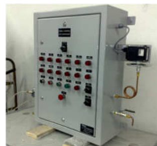
Vista externa - Painel p/ EGSA
